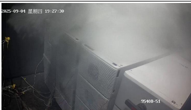
Figure 2.30: During 5 th cell (cell 7) thermal runaway (Local Time in 19:27)
