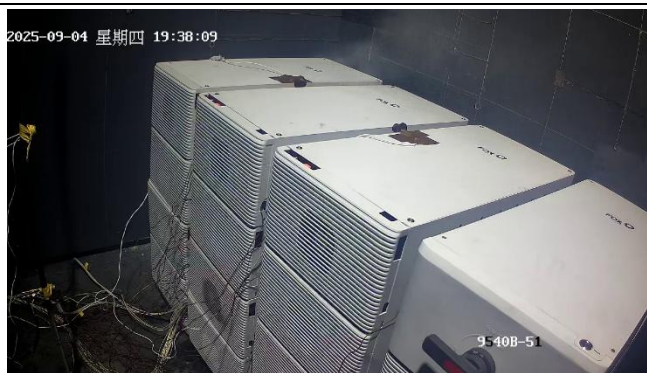
Figure 2.32: During 6 th cell (cell 8) thermal runaway (Local Time in 19:38)
