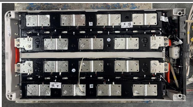
Figure 2.7: Internal view of initiating module-2
