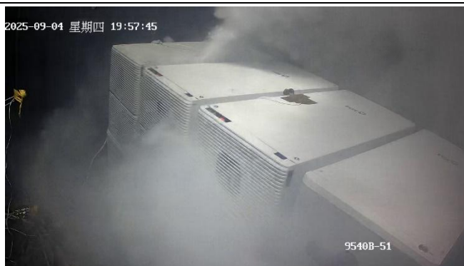
Figure 2.33: During 6 th cell (cell 8) thermal runaway (Local Time in 19:57)
